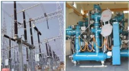
AIS / GIS Sub-station
