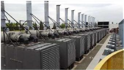
Data Centre Infrastructure
